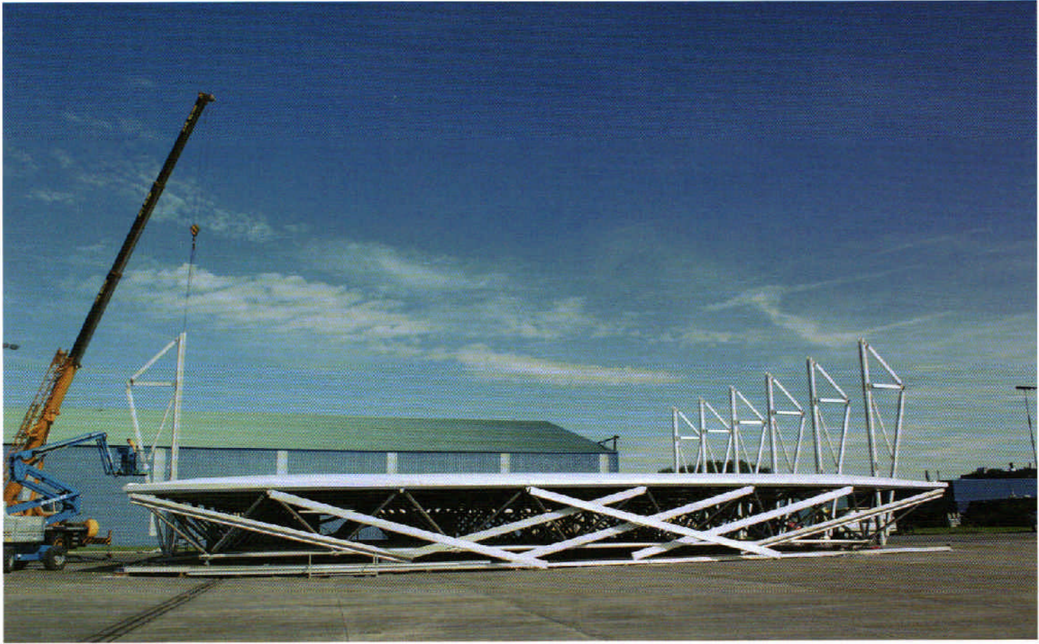
The temporary front of house facilities under construction Photo: Joris van Bennekom
